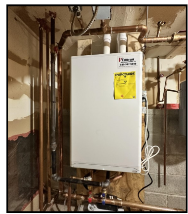
Our New Boiler
