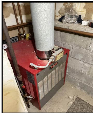
Our Old Boiler
