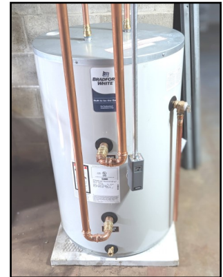
Hot Water Tank
