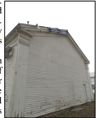
Fellowship Hall Damaged During Wind Storm
