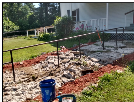
Church Sidewalk Needing Repair
