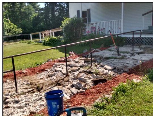
Church Sidewalk Needing Repair
