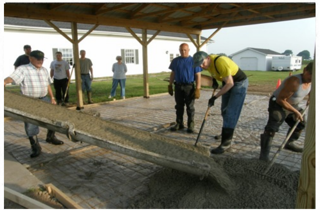
Men at Olcott Bible Church Pour Concrete Pad in Wood Storage Facility
